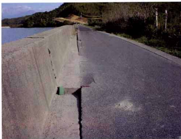
写真-18 護岸の損壊
